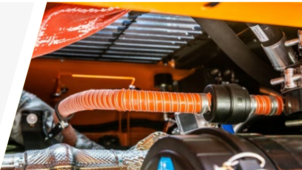
Heavy-duty filtration system (ejector)
